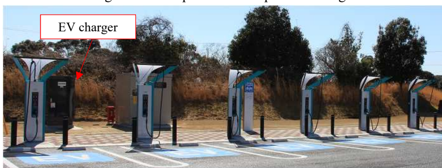
Figure 2: Example of a multi-port EV charger
